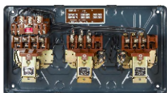
Interior View of MK2 SASD
