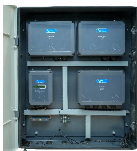
Interior View of xMasm10 - Wired Solution
