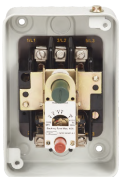
Interior View of MF1 DOL - 3Ø Starter
